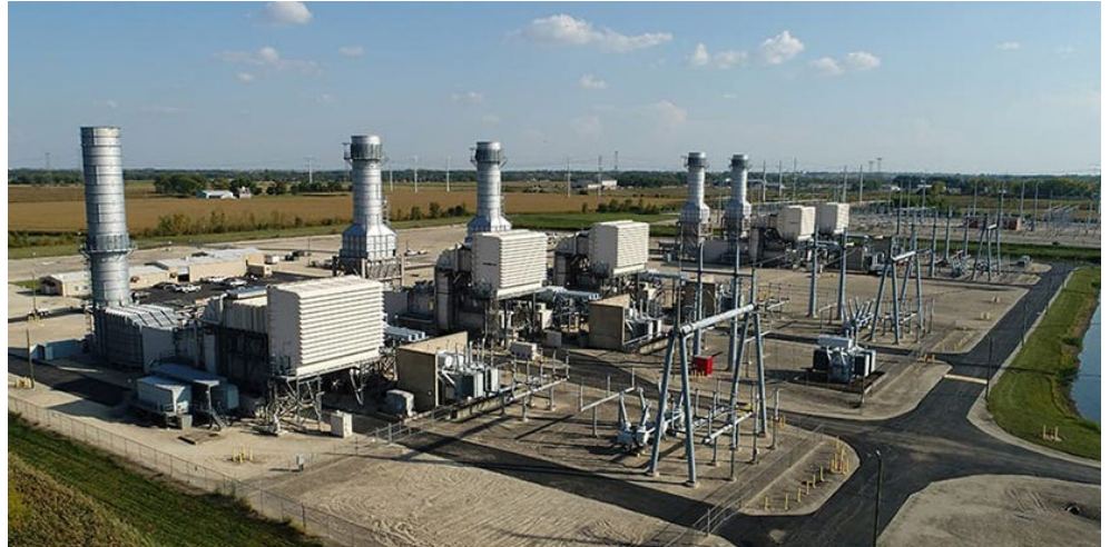
J-Power's Elwood Energy Center, a 1,350-MW natural gas turbine in Illinois | J-Power
