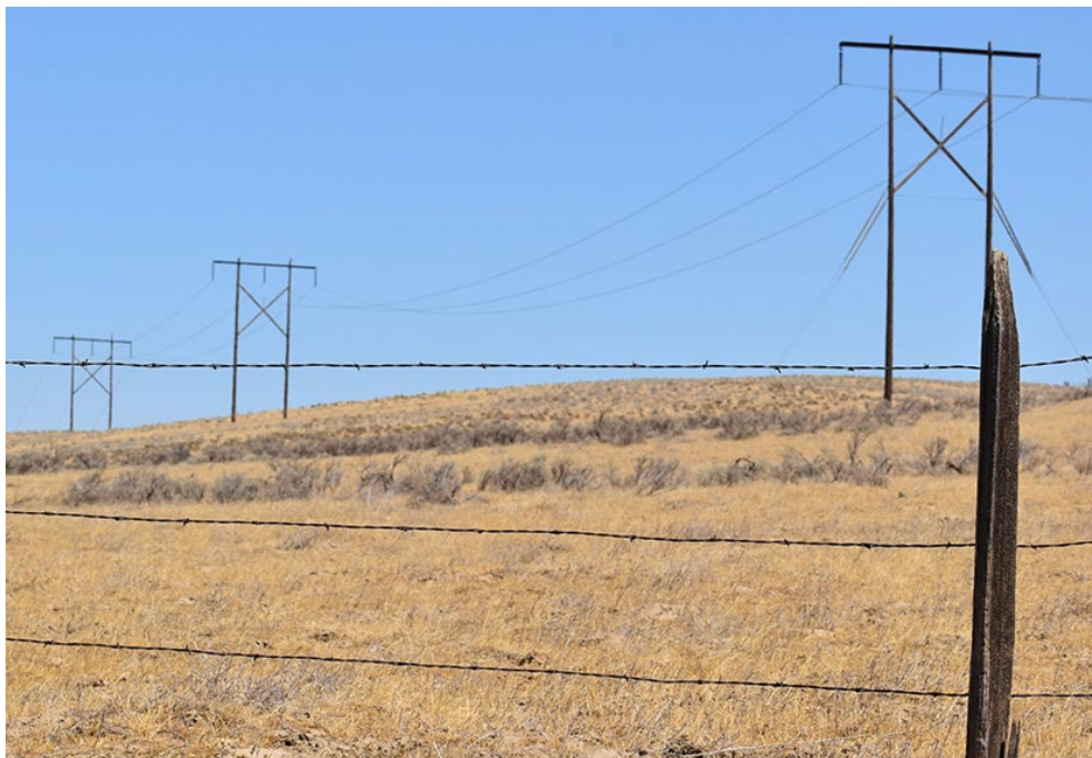
BPA transmission line in Umatilla County, Ore. | © RTO Insider LLC
