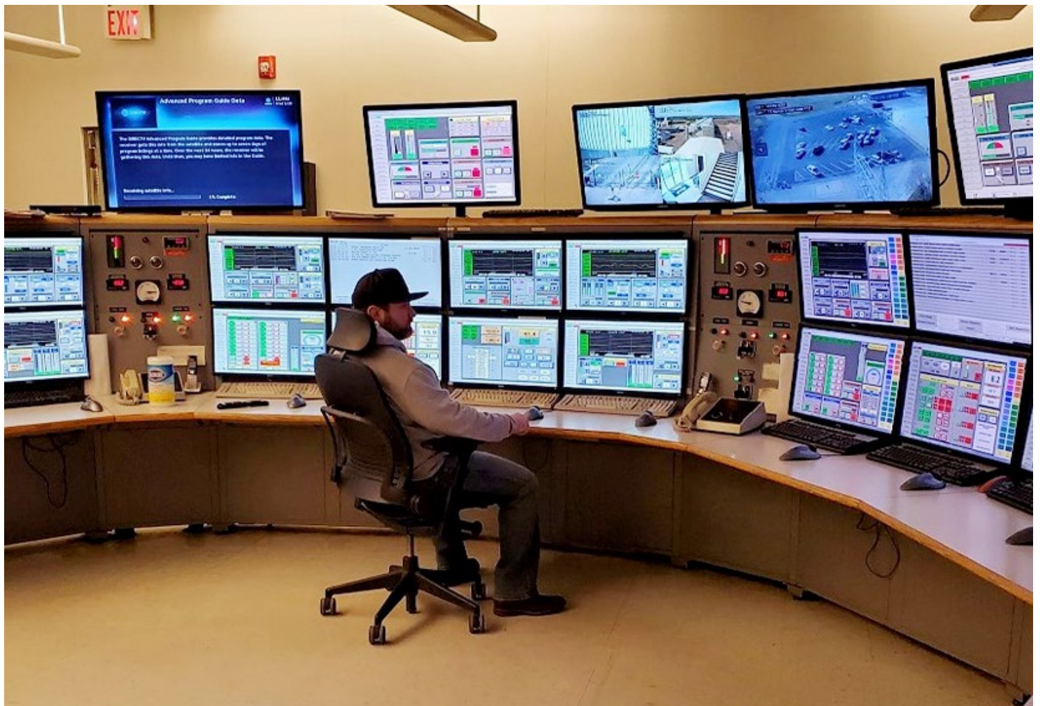
An Xcel Energy control room | Xcel Energy
