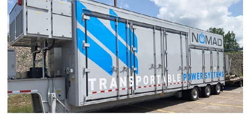
Green Mountain Power's mobile 2-MWh battery system | Green Mountain Power
