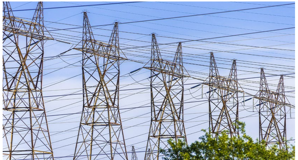
Transmission lines near Niagara Falls are shown. The New York Public Service Commission has adopted a coordinated grid planning process to expedite expansion of transmission capacity. | Shutterstock
