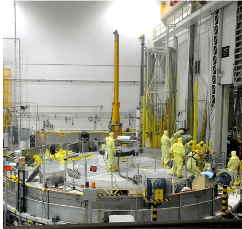
Maintenance and refueling is performed at the Idaho National Laboratory’s advanced test reactor. | Idaho National Laboratory
