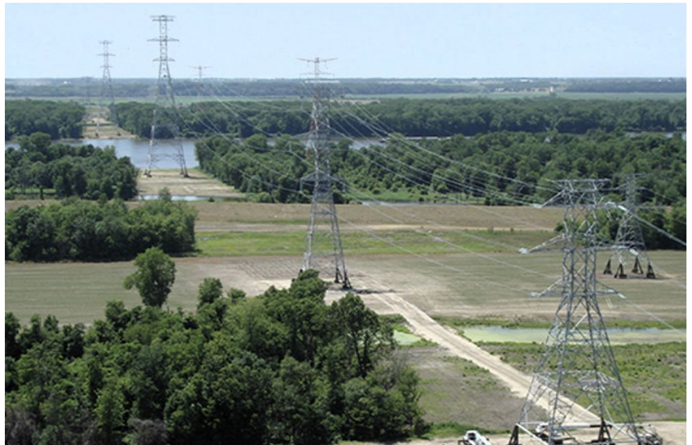
Ameren Illinois Rivers Transmission Project | Hanson Professional Services
