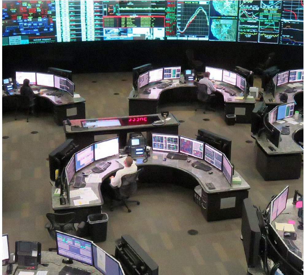
CAISO's control room in Folsom, Calif. | CAISO
