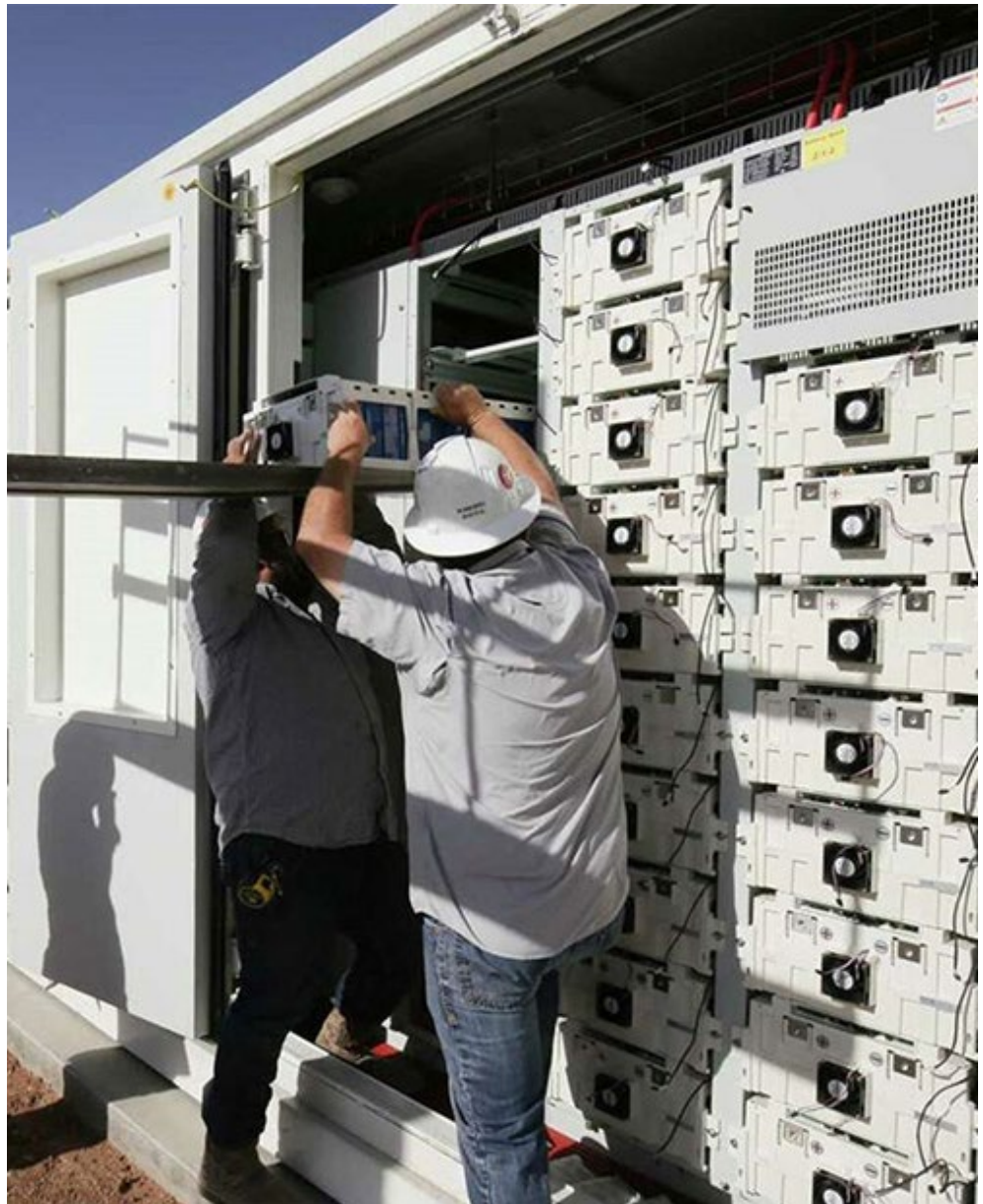
A Broad Reach Power crew works on a storage facility in West Texas. | Broad Reach Power
