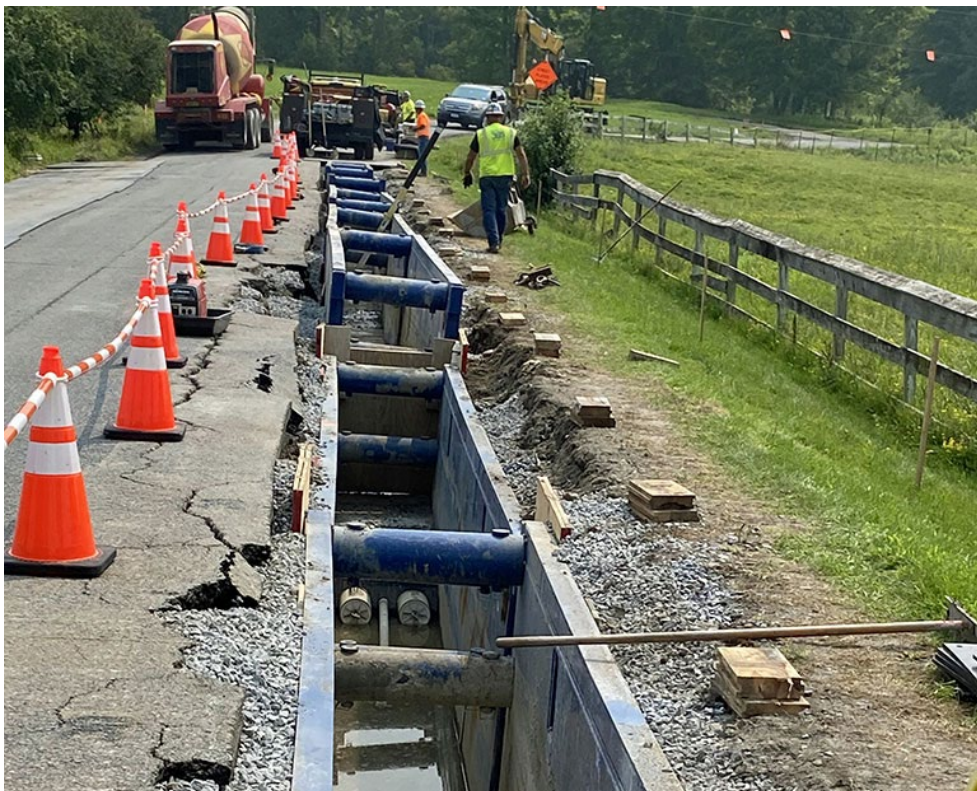
Work on the Champlain Hudson Power Express near Lake Champlain recently | NYSERDA
