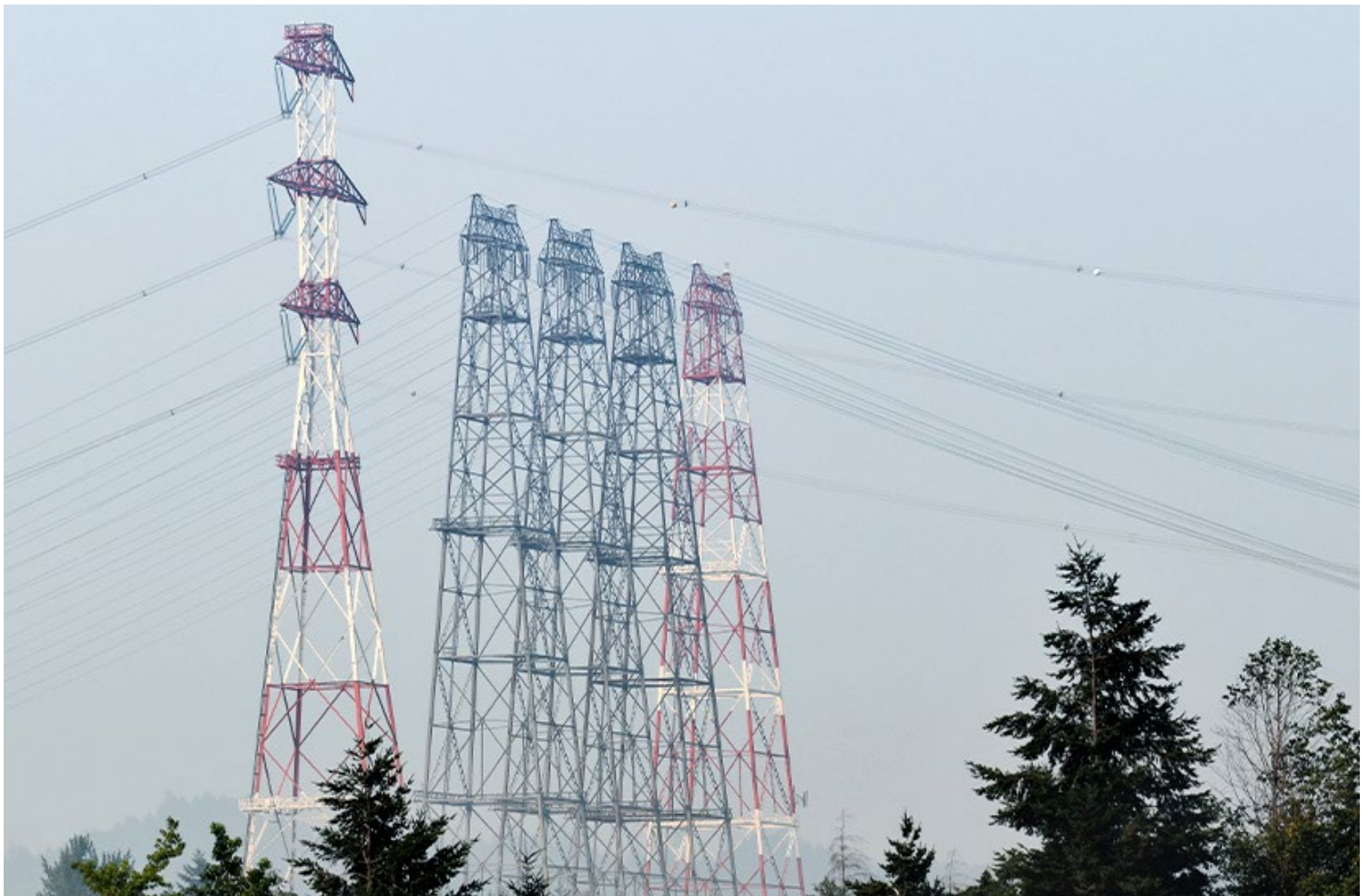
BPA transmission line near the Bonneville Dam | © RTO Insider LLC
