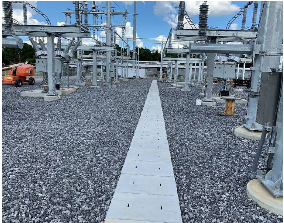
Entergy Mississippi substation | Malouf Construction
