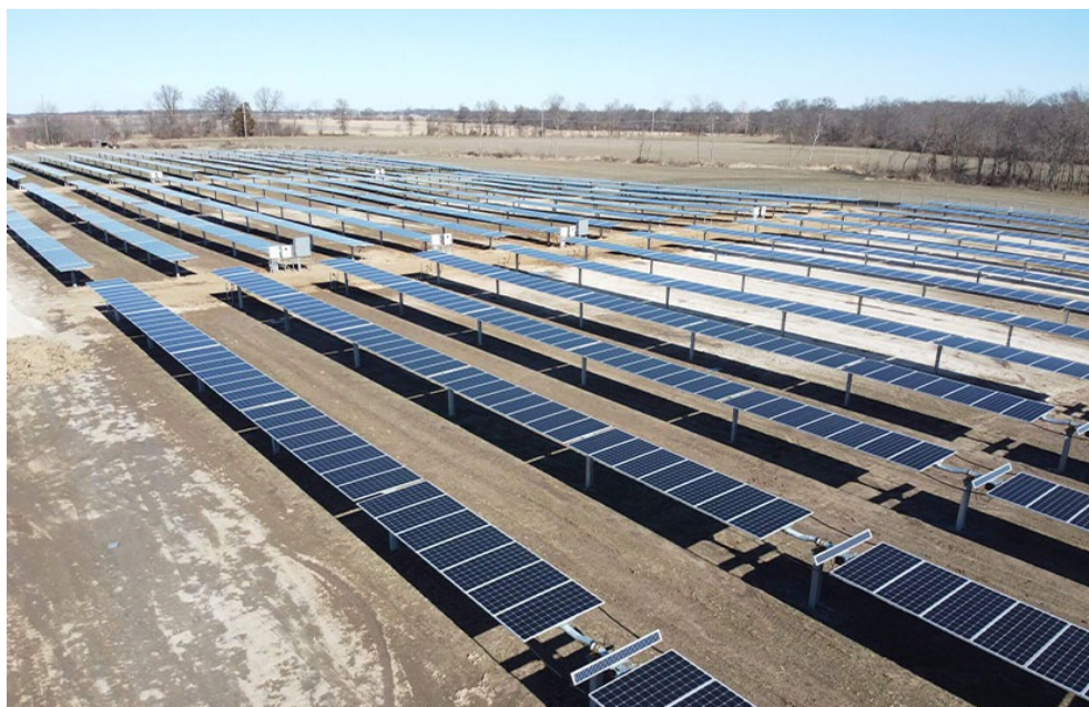
EDF Renewables' Sandoval solar project in Illinois was completed in 2021. | Solstage
