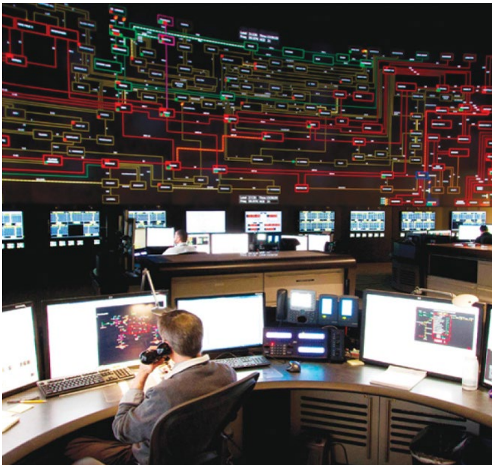
NYISO control room in Rensselaer, N.Y. | NYISO
