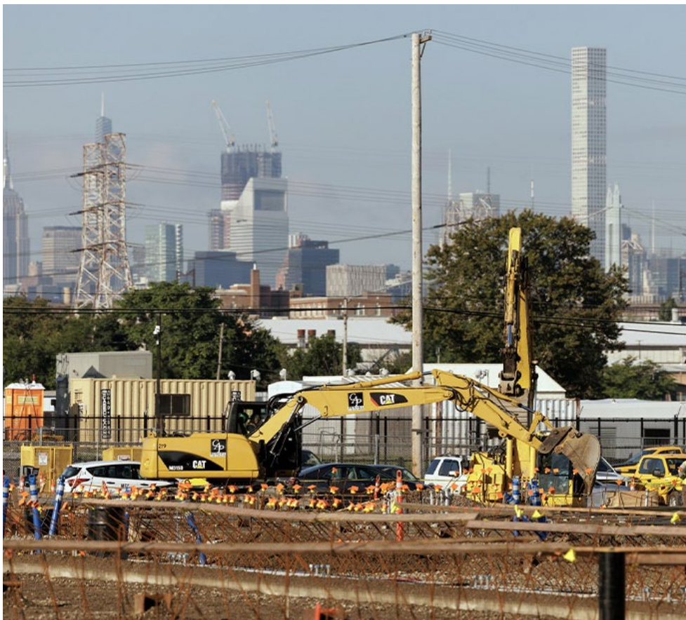
Work is shown Sept. 19 on the Champlain Hudson Power Express converter station in New York City. | New York Governor's Office
