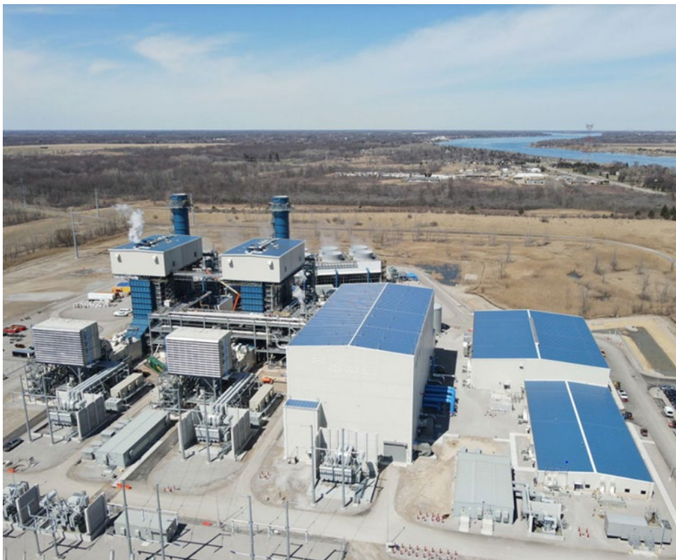
Construction of DTE Energy's natural gas-fired Blue Water Energy Center in 2022 | DTE Energy
