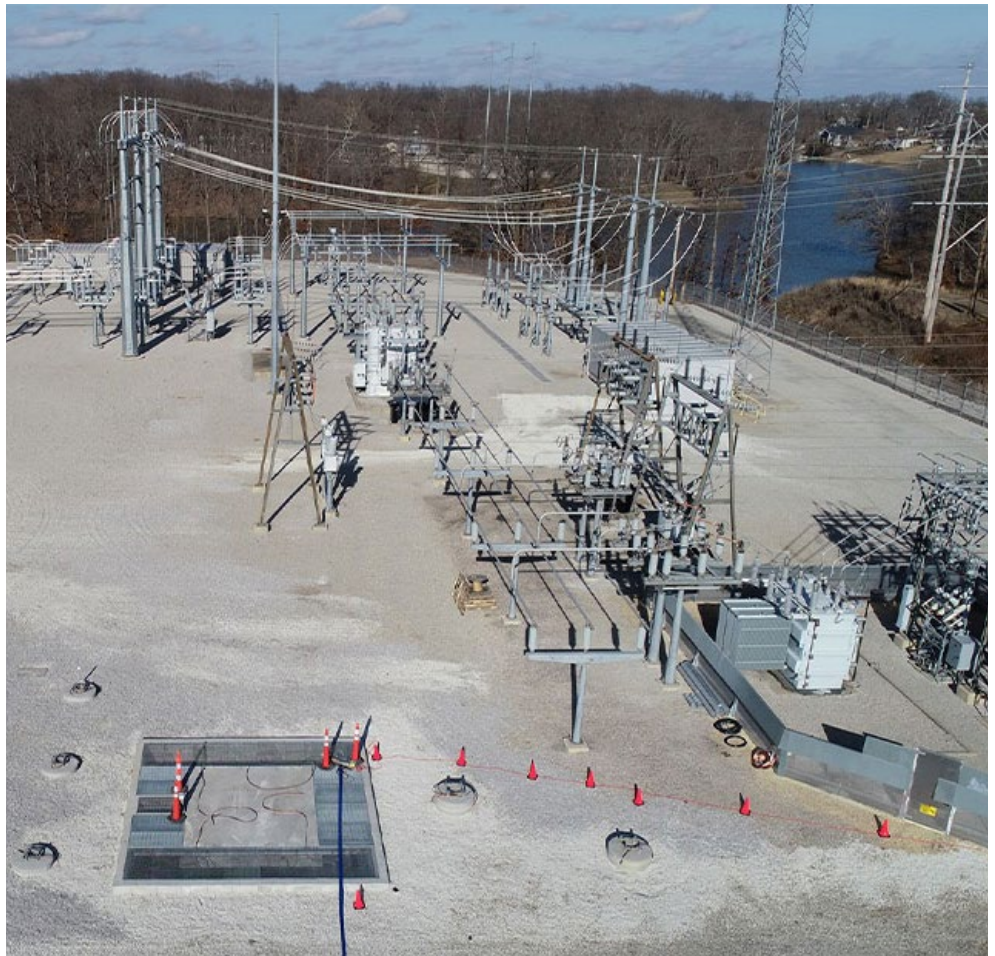
An Ameren Illinois substation expansion in 2021 | Ameren Illinois
