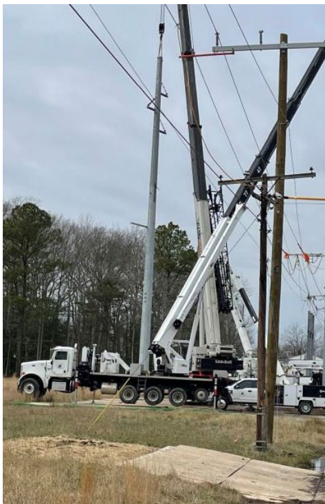
During Exelon's Q3 earnings call, CFO Jeanne Jones highlighted Delmarva Power's $40 million East New Market to Cambridge grid upgrade project on Maryland's Eastern Shore. | Delmarva Power & Light
