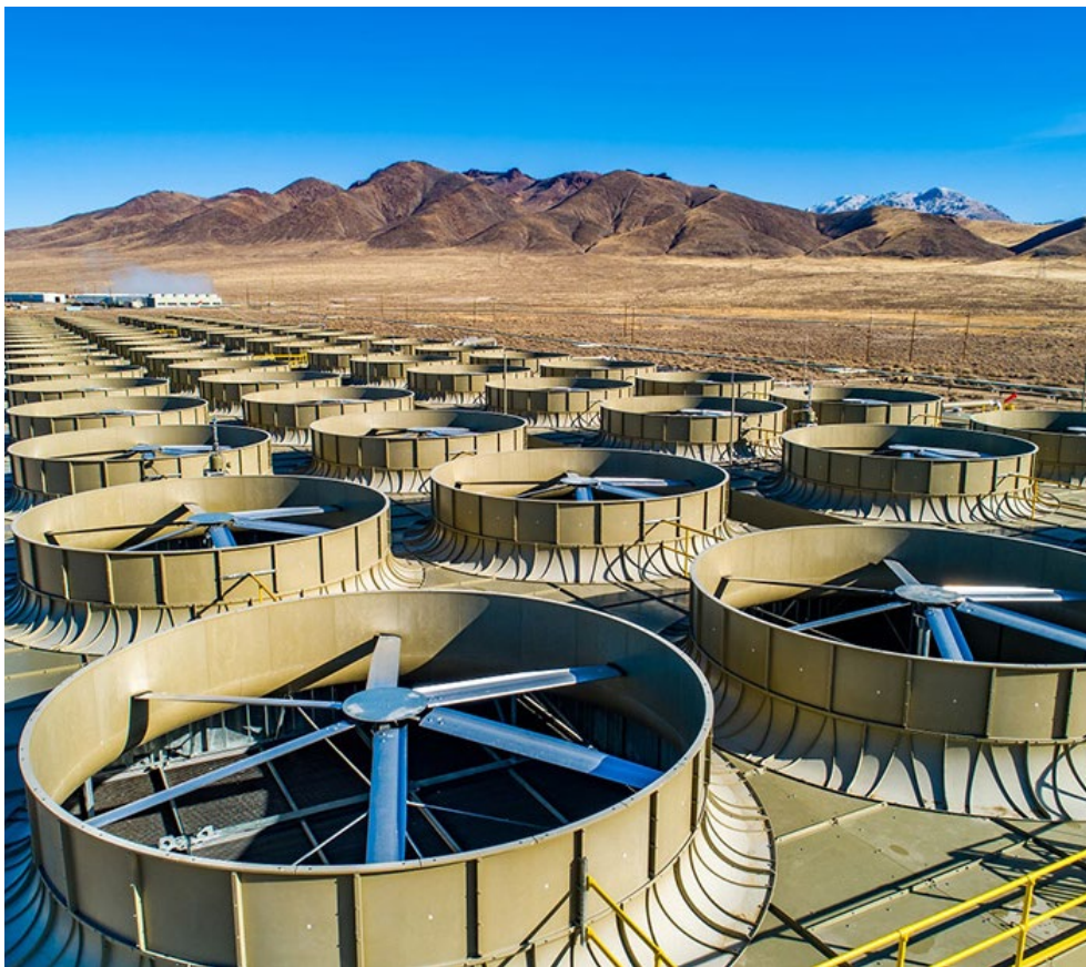
Ormat Technologies, which recently completed the North Valley geothermal power plant in Nevada, was the winning bidder for five Nevada geothermal parcels that the BLM auctioned this week. | Ormat Technologies
