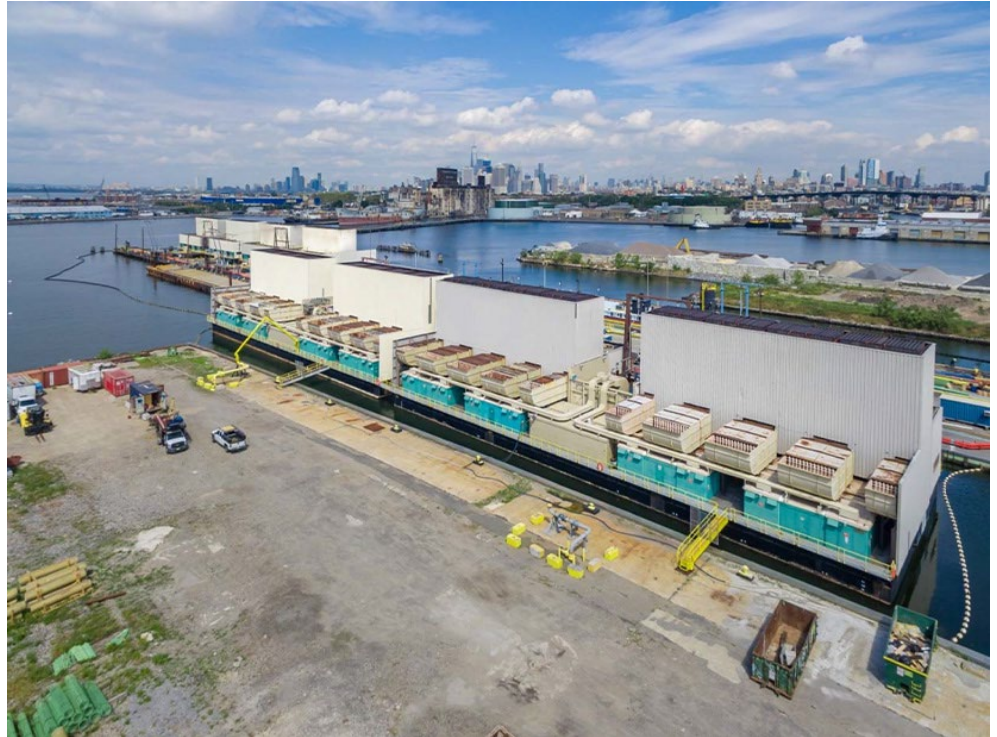
Gowanus barge-mounted natural gas generating station in Brooklyn, New York | Astoria Generating Company
