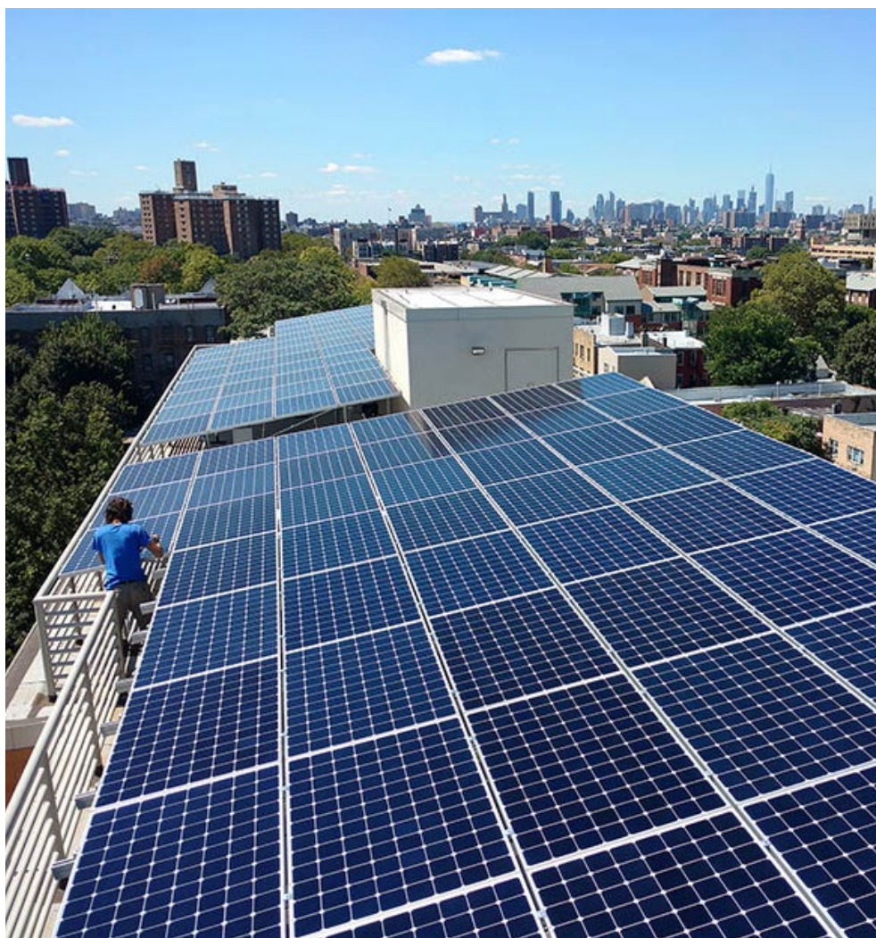
Solar panels on a rooftop in New York City | Bright Power, Inc.
