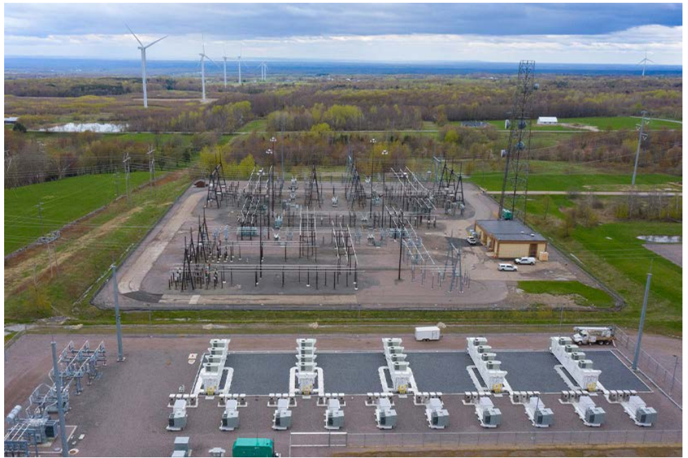
The New York Power Authority’s new Northern New York Energy Storage Project is shown in May 2023. | NYPA
