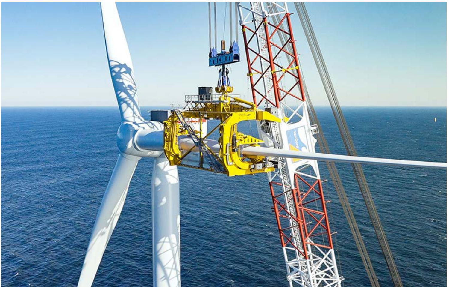
The first turbine blades are attached at the South Fork Wind Project, the first offshore wind farm powering New York. | South Fork Wind
