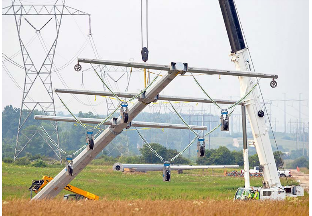
Work progresses on the New York Power Authority's Central East Energy Connect transmission upgrade. | NYPA
