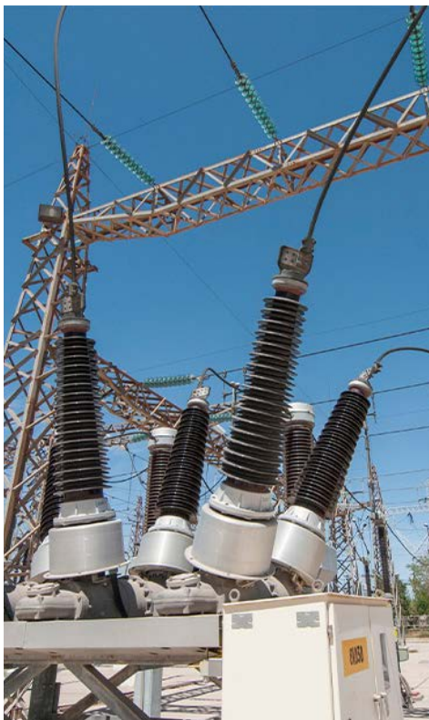
Sulfur hexafluoride equipment is shown at a geothermal power plant substation. New York is proposing new regulations on SF6, the most potent greenhouse gas. | Shutterstock
