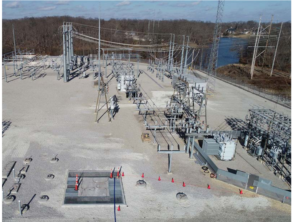
An Ameren Illinois substation expansion in 2021 | Ameren Illinois
