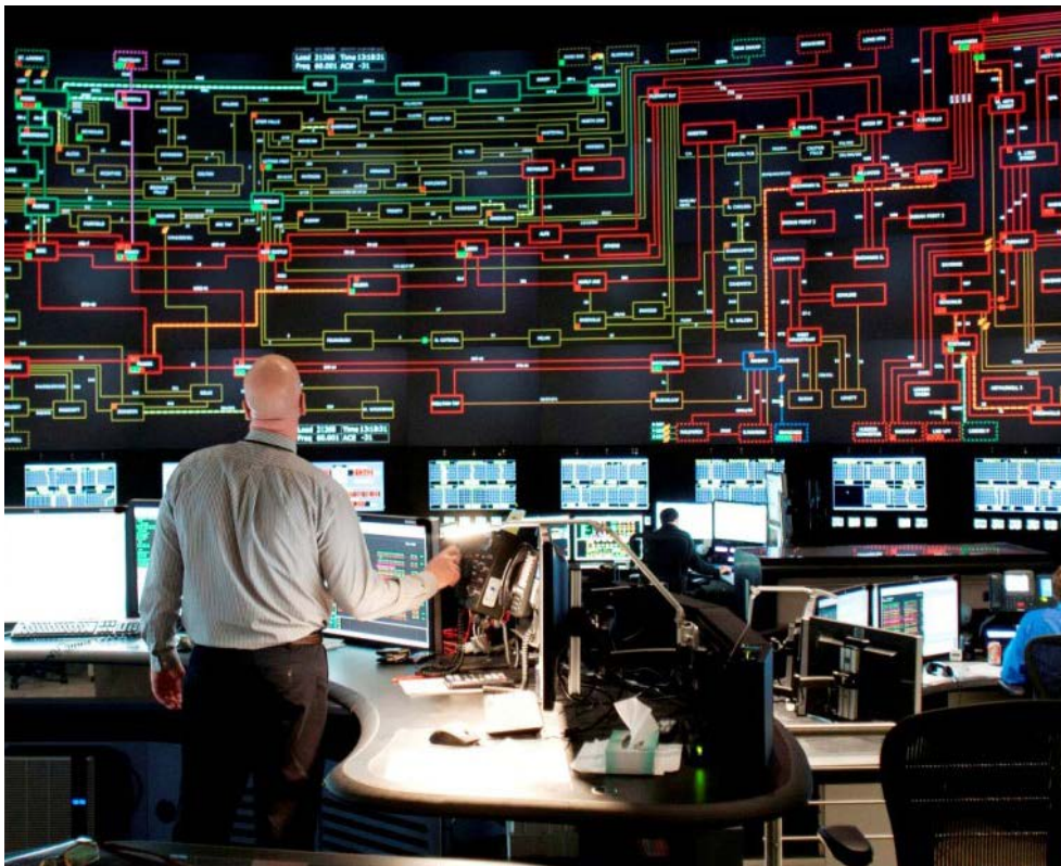
NYISO control room in Albany, N.Y. | NYISO
