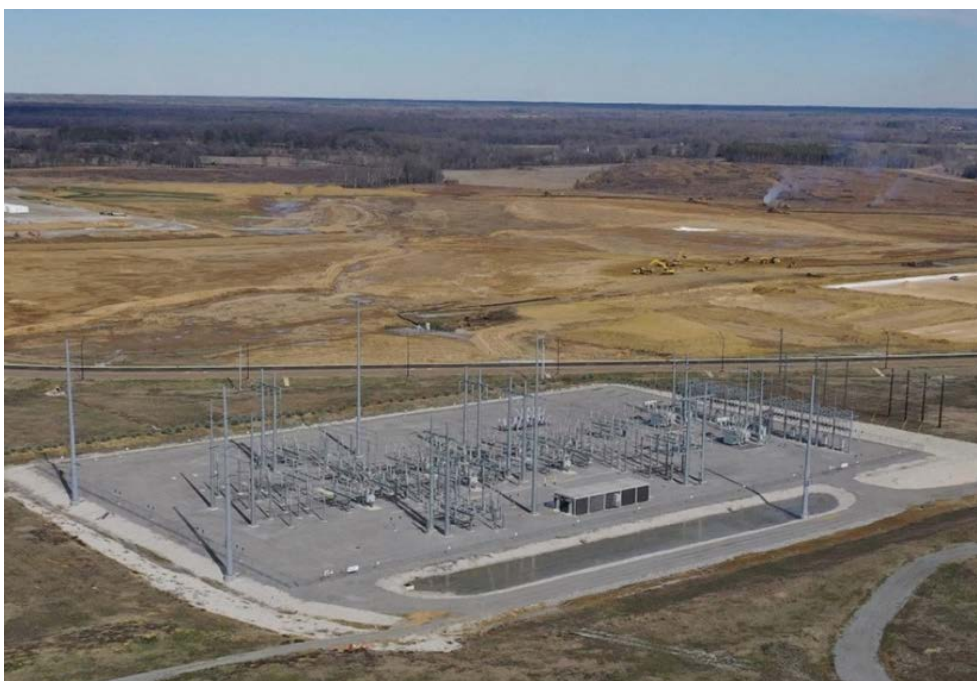
A future Amazon data center megasite on the campus in Madison County, Mississippi | Entergy
