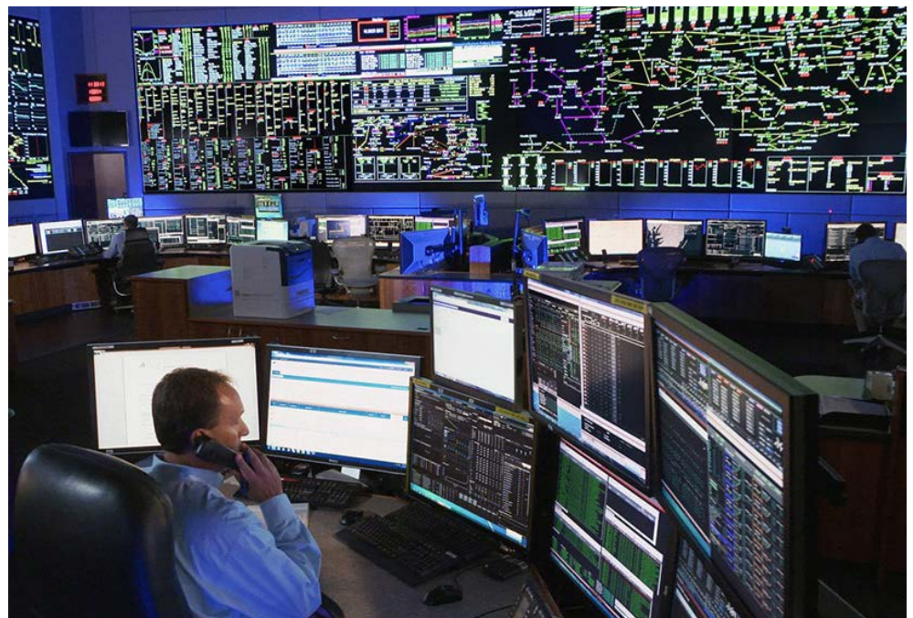
PJM control room | PJM
