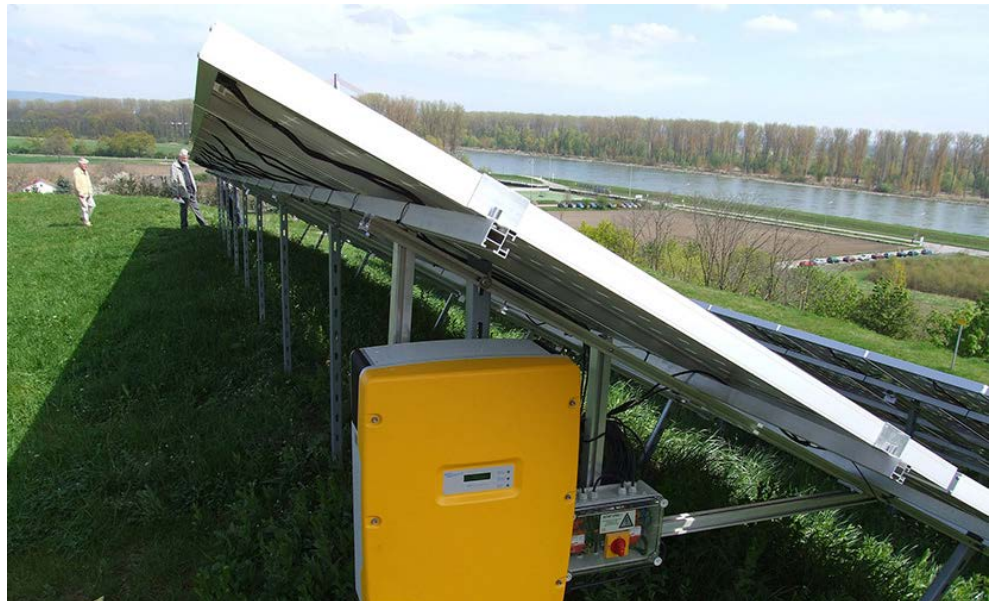
Inverter-based resource with electronic power converter | Claus Ableiter, CC BY-SA 3.0, via Wikimedia Commons
