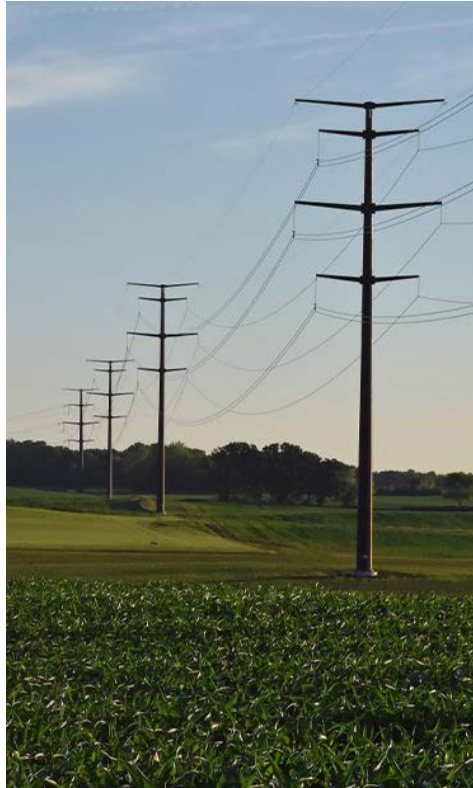
A 345-kV MISO multivalue project ITC Midwest completed near the Iowa-Minnesota border in 2017 | ITC Midwest
