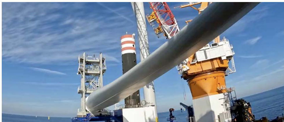
Construction work continues on South Fork Wind. Eversource has reached a deal to divest its interest in South Fork and other offshore wind projects. | South Fork Wind
