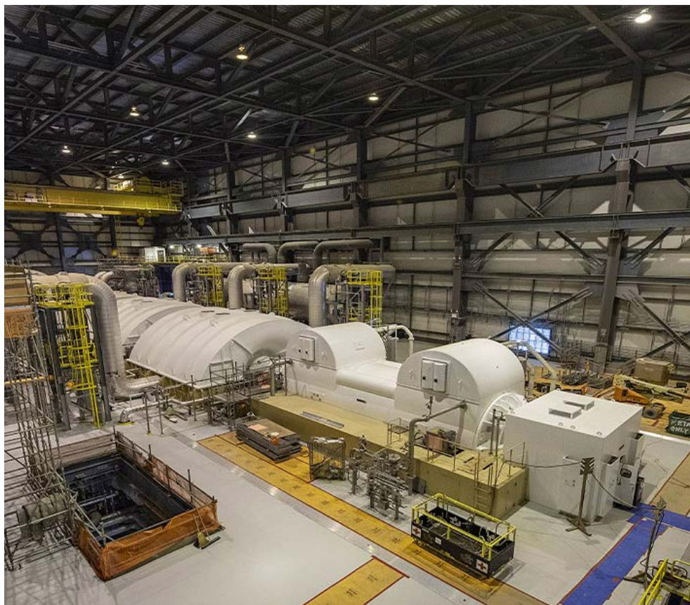
The turbine generator at Unit 4 of the Vogtle nuclear power plant in Georgia, which achieved initial criticality on Feb. 14. | Georgia Power
