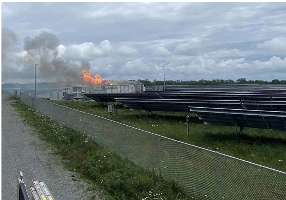
A battery energy storage system fire burns near Chaumont, N.Y., in July 2023. | Three Mile Bay Fire Company
