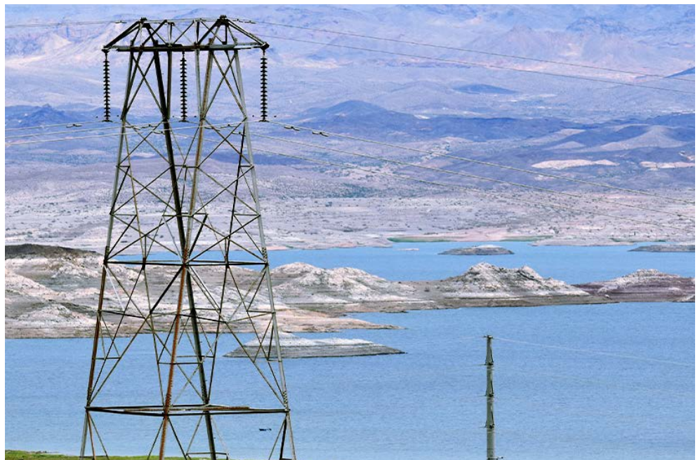
Transmission line near Lake Mead in Nevada. | © RTO Insider LLC
