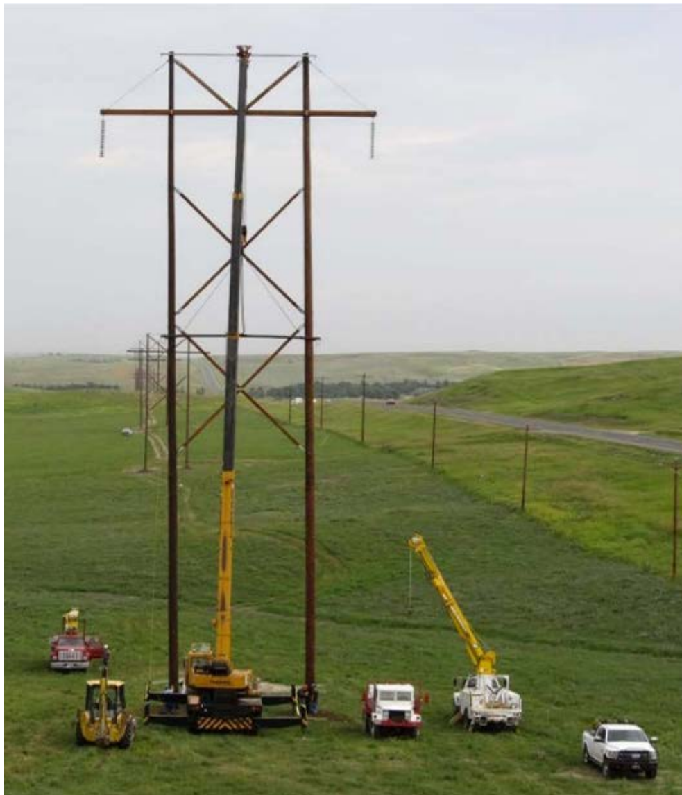
Transmission construction near the Charlie Creek flowgate area | Western Area Power Administration
