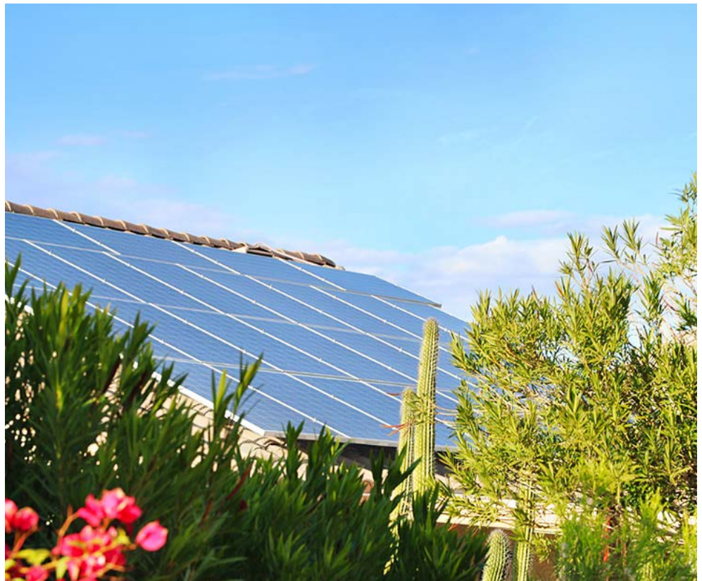
| Sun Valley Solar Solutions
