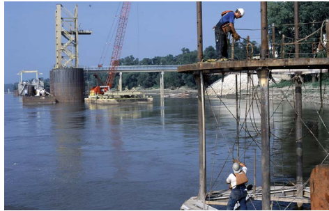
Construction on a coal unloading facility for Ameren's Rush Island Power Plant in 2020. | Massman Construction Co.
