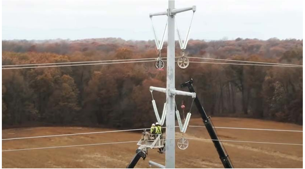
Construction on ATXI's Mark Twain transmission line in Northeast Missouri | IBEW Local 2
