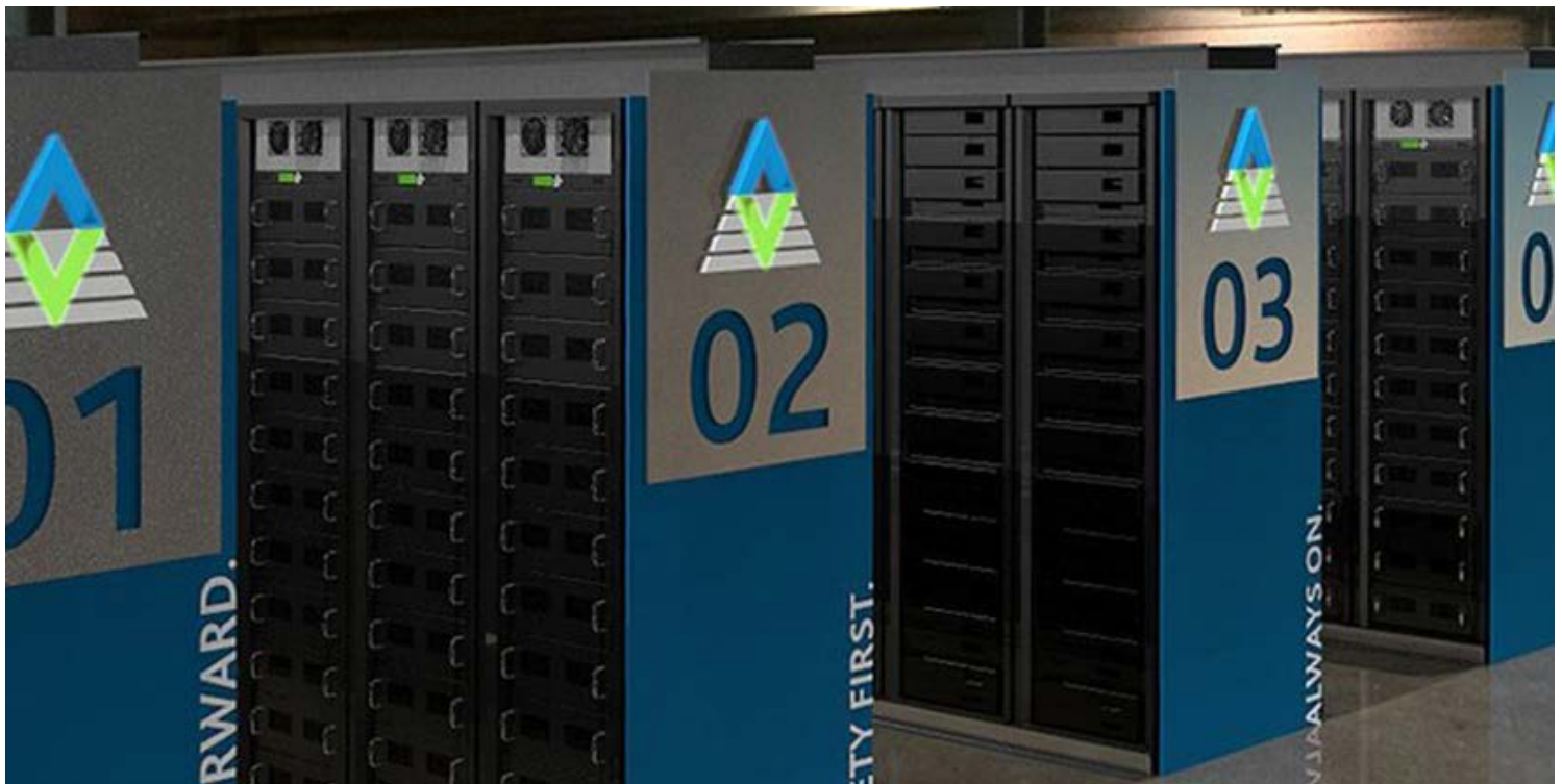
The interior of AES Indiana's Advancion battery storage array, which has been operating since 2016 at its Harding Street Station | AES Indiana
