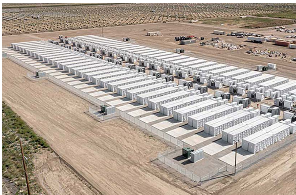
RWE battery storage facility in Fresno County, Calif. | RWE
