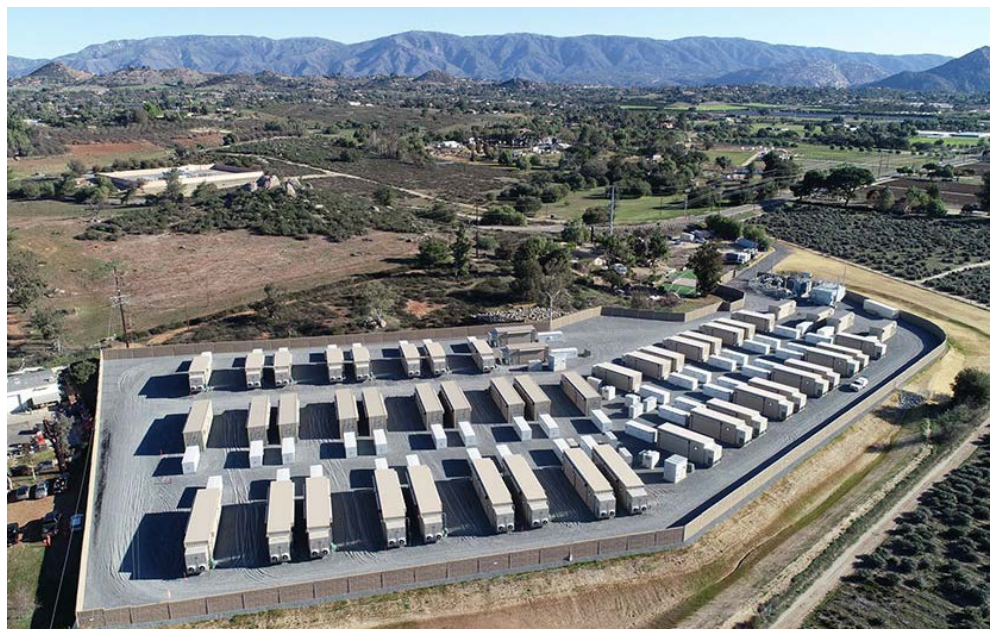
Terra-Gen's Valley Center energy storage facility in San Diego County, Calif. | Terra-Gen
