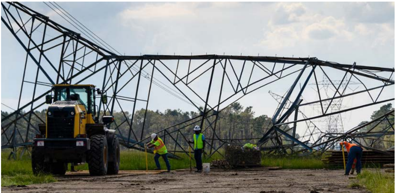
Damage to Entergy's transmission system as a result of Hurricane Laura in 2020 | Entergy
