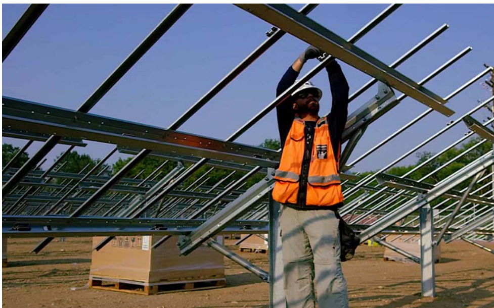
Construction of a Michigan solar farm for Consumers Energy | National Grid Renewables
