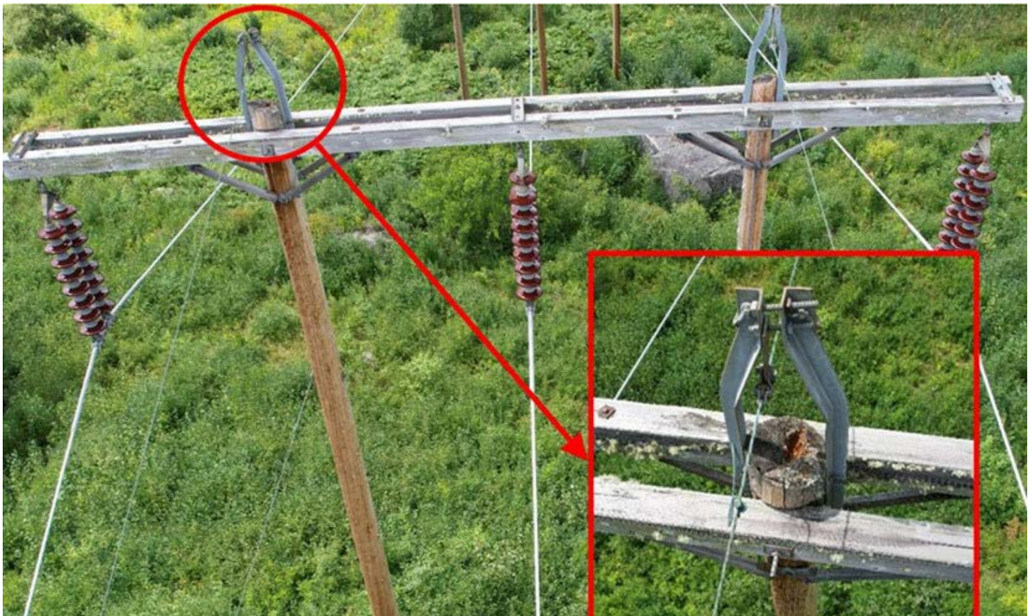
Pole deterioration on Eversource's X-178 Line in New Hampshire | Eversource
