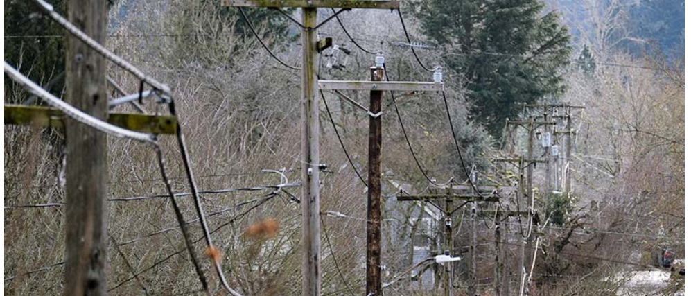
PGE distribution lines in Portland, Ore. | © RTO Insider LLC
