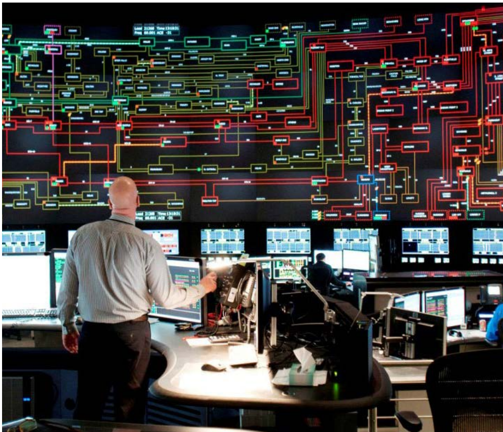
NYISO control room in Rensselaer, N.Y. | NYISO
