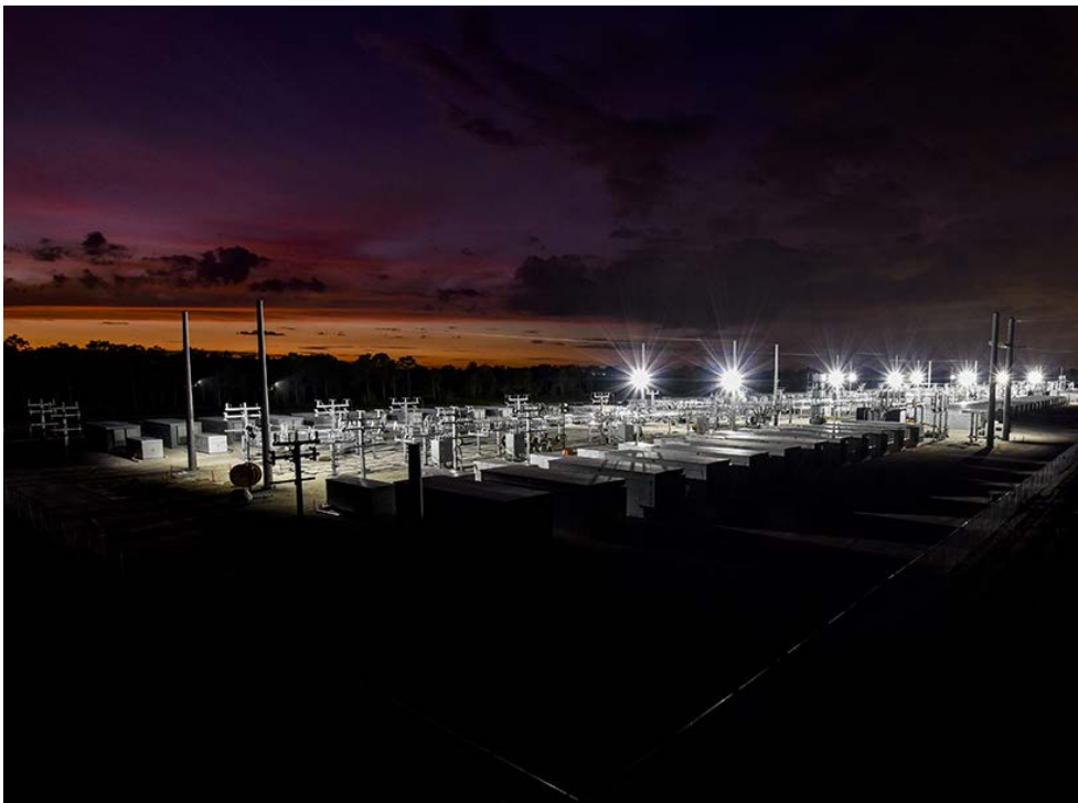
PPL's Manatee Energy Storage Center is shown in Parrish, Fla. | NextEra Energy
