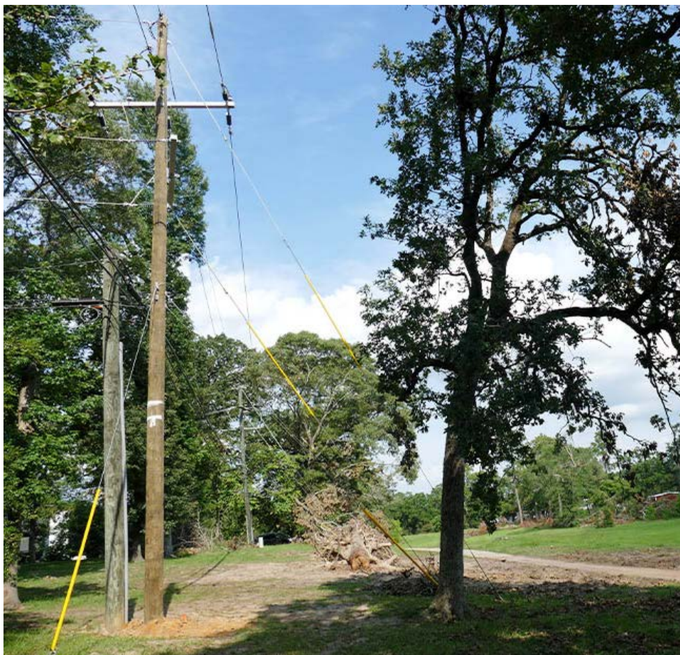
New utility poles line right-of-way amid the storm’s debris in Conroe. | © RTO Insider LLC
