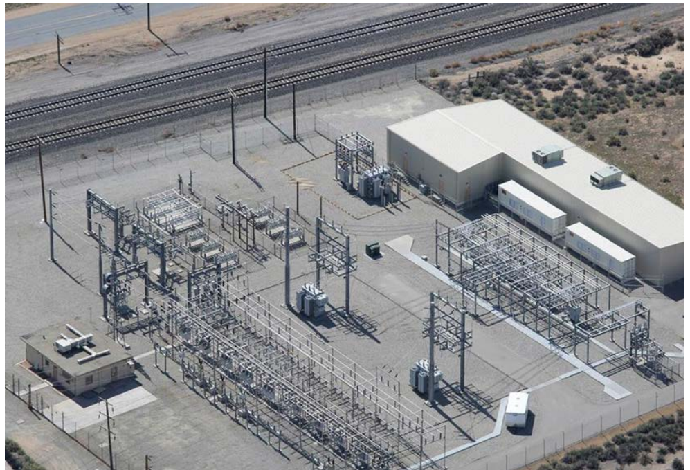
View of the Tehachapi Energy Storage Project in Tehachapi, Calif. | Sandia National Laboratories
