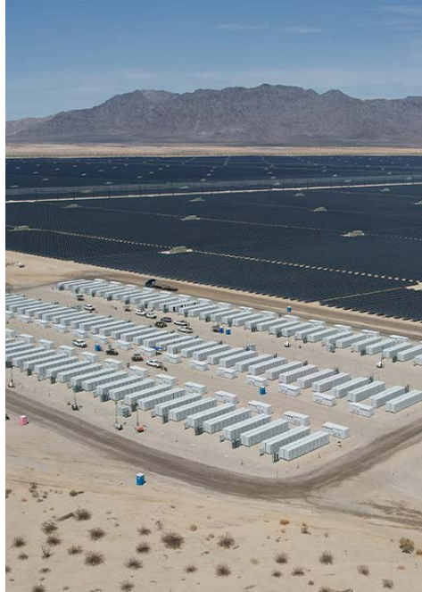
The 230-MW Desert Sunlight Battery Energy Storage System in Riverside County, Calif. | Bureau of Land Management California
