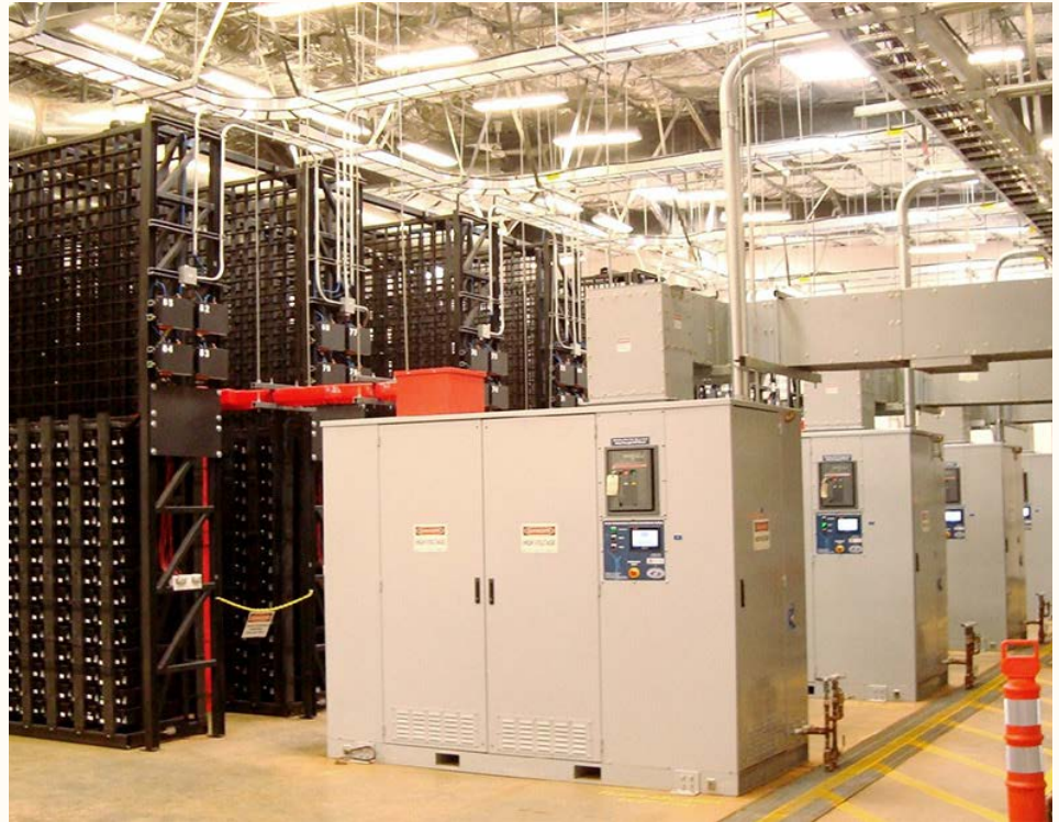
Kahuku battery storage facility in Hawaii | Mike Jacobs
