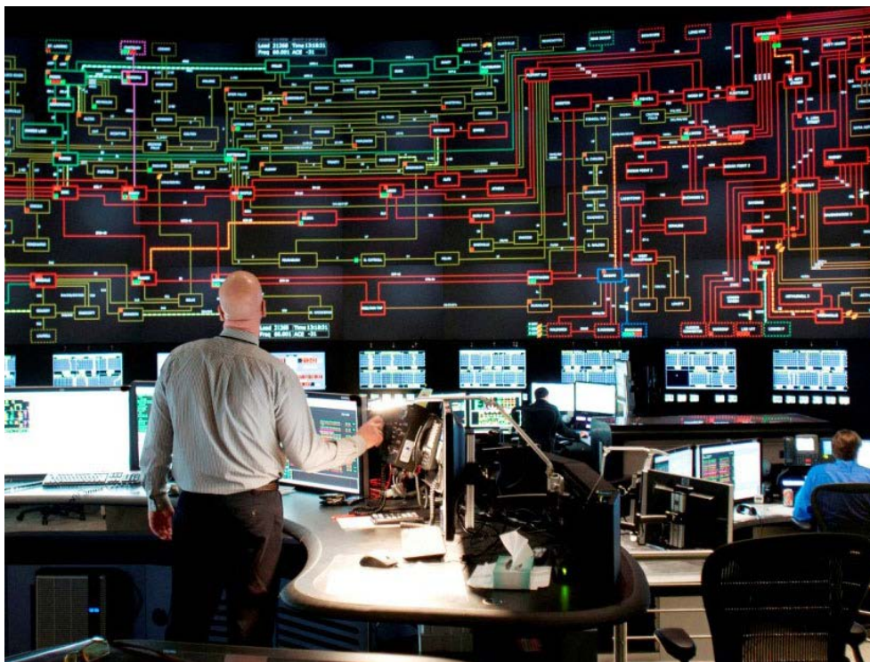
NYISO control room in Rensselaer, N.Y. | NYISO
