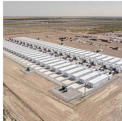
Fifth Standard, RWE Clean Energy’s first utility-scale battery storage project in California. | RWE
