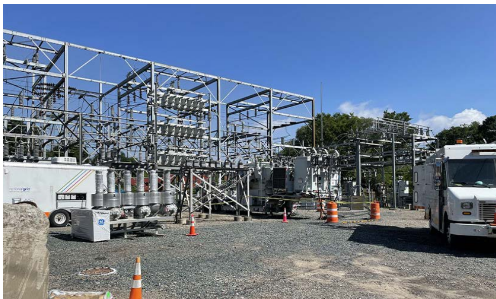
Upgrades are shown in progress at the National Grid substation in Gloversville, N.Y. | National Grid
