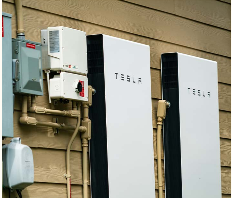
Tesla Powerwall batteries | Shutterstock
