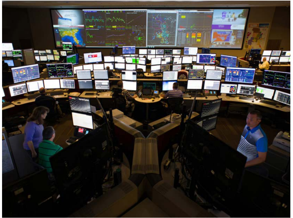
SPP's control room | SPP
