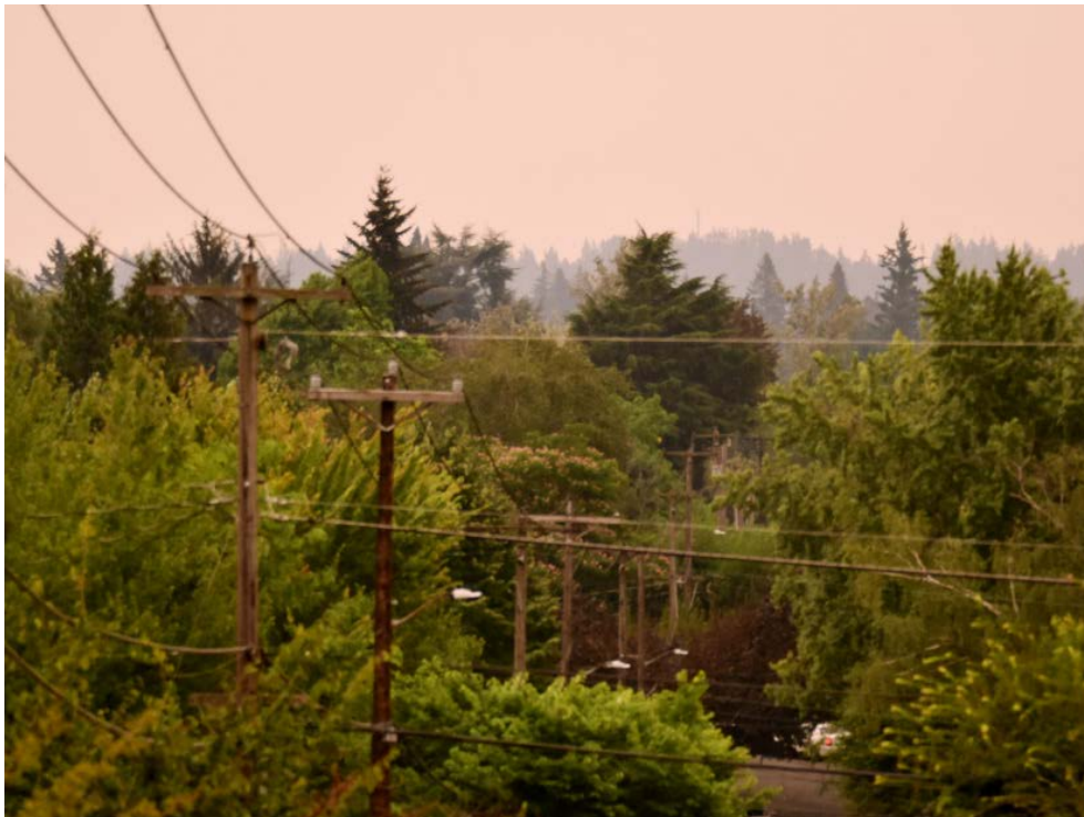
PGE distribution lines in Portland, Ore. | © RTO Insider LLC
