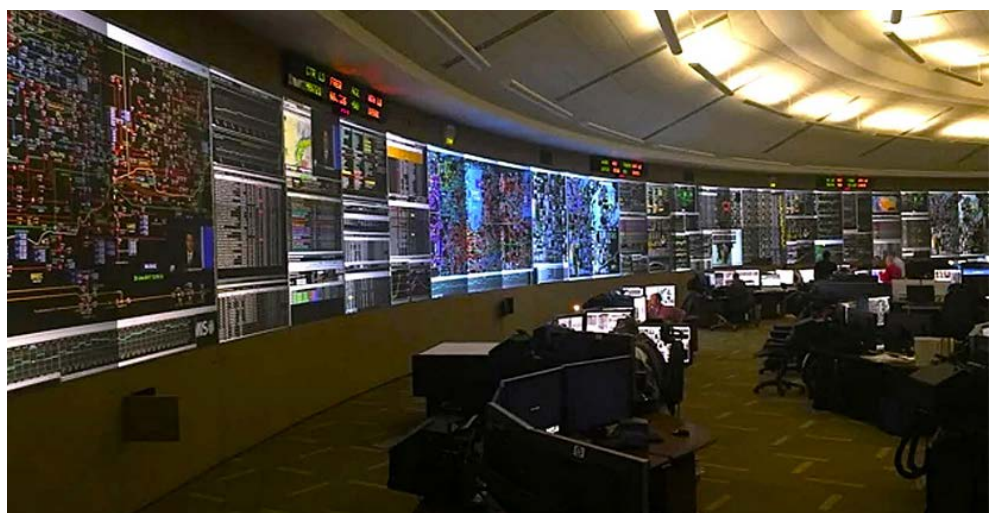
MISO control room | MISO
