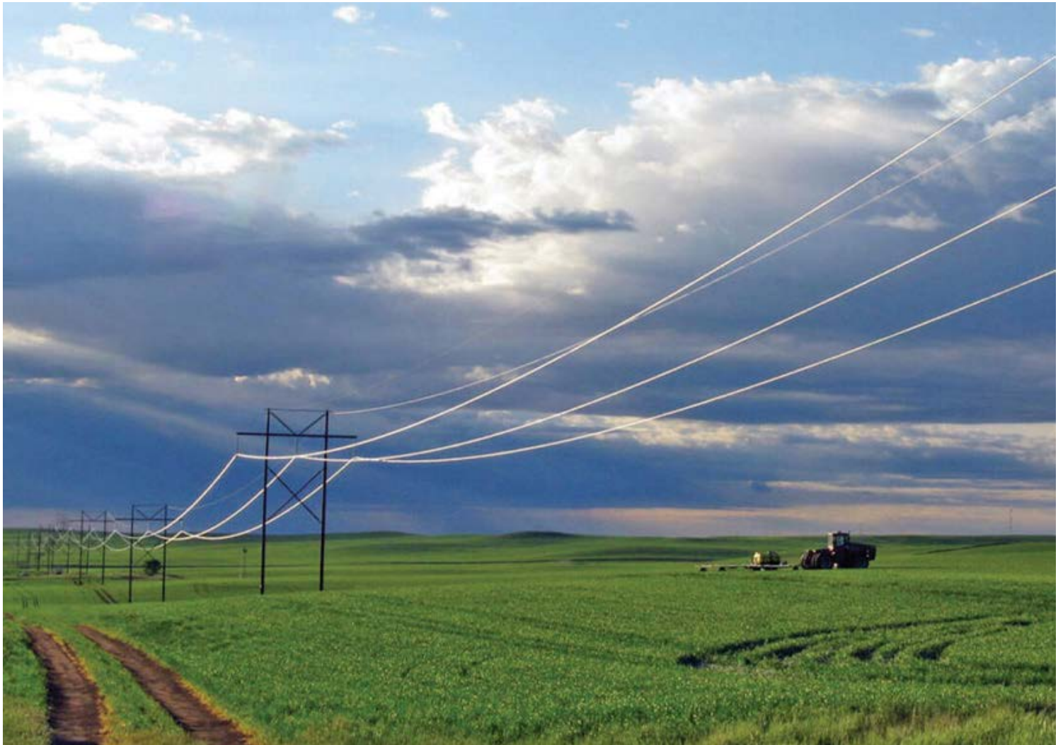
Line in Williston, N.D. | Western Area Power Administration
