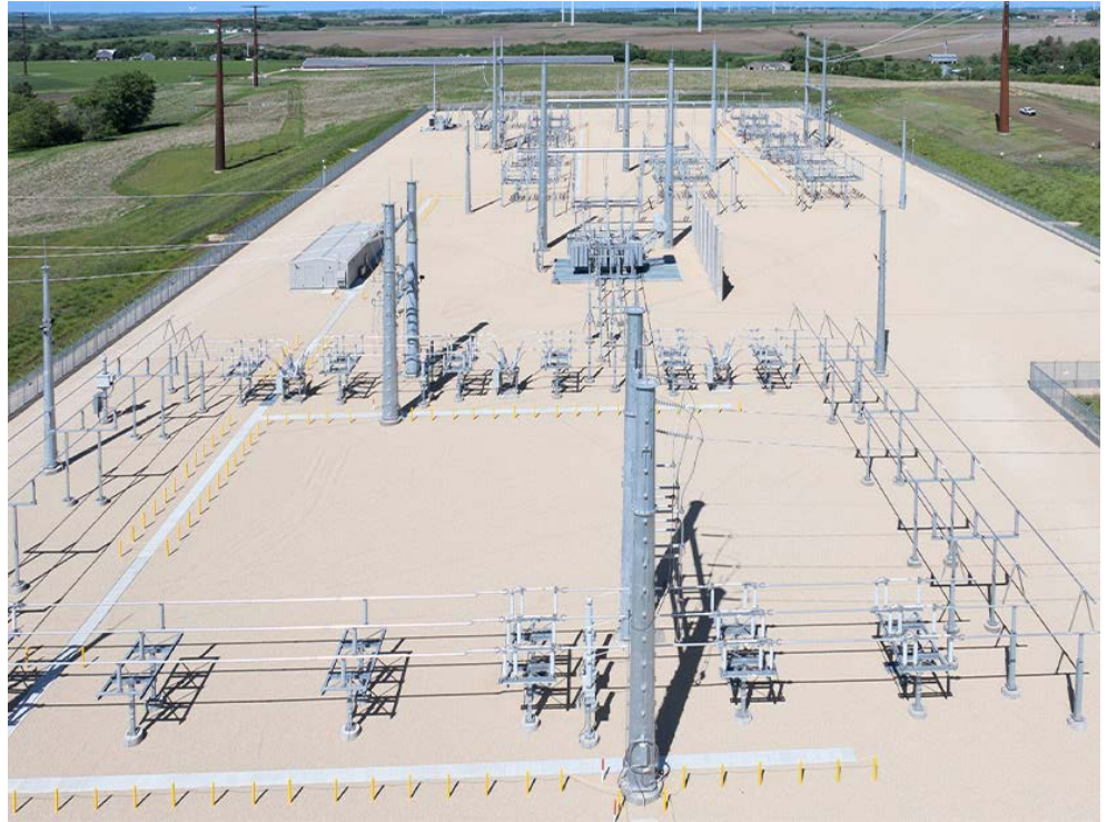
Hill Valley substation, completed as part of the Cardinal-Hickory Creek line in Wisconsin | ITC and ATC
