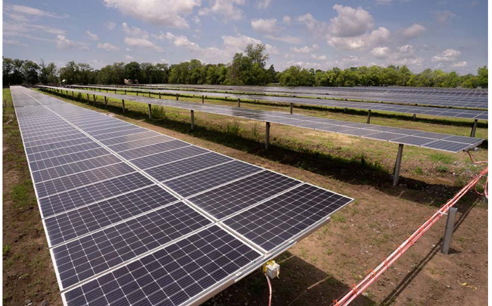
Capital Region Solar in West Baton Rouge Parish | Entergy Louisiana
