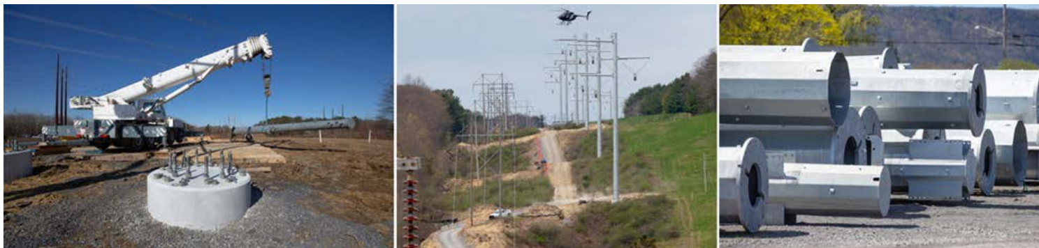
A collage of images from the New York Power Authority showing initial construction of the Central East Interconnection transmission upgrades. | NYPA
