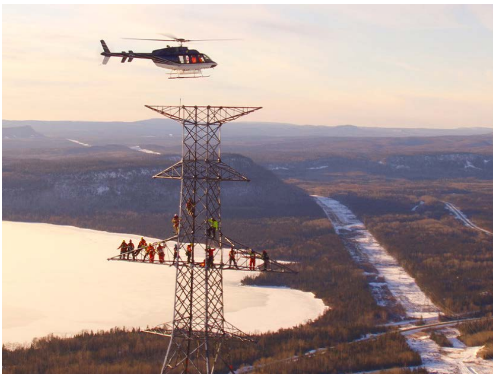
The East-West Tie is shown under construction in Ontario. NextEra Energy Transmission Canada is a partner. | NextEra Energy
