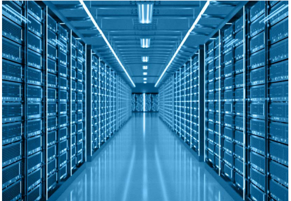
Xcel Energy says data center load will accelerate its ability to develop both transmission and generation. | Ascenty
