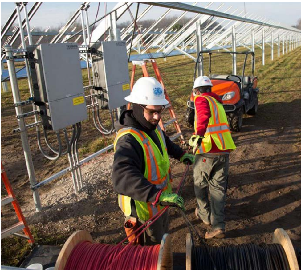
Solar array installation in Michigan for Wolverine Power Cooperative | J. Ranck Electric
