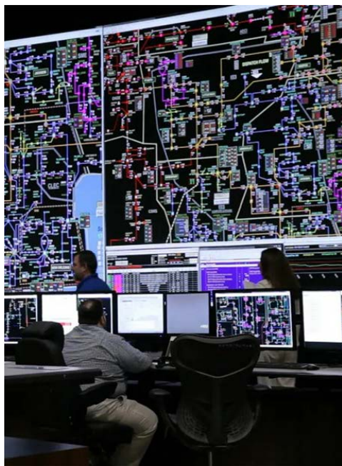
MISO control room | MISO
