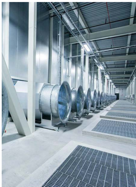
Cooling fans in a Meta data center | Meta
