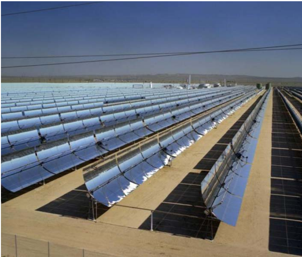
Sonoran West Solar Holdings in Riverside County, Calif. | NREL
