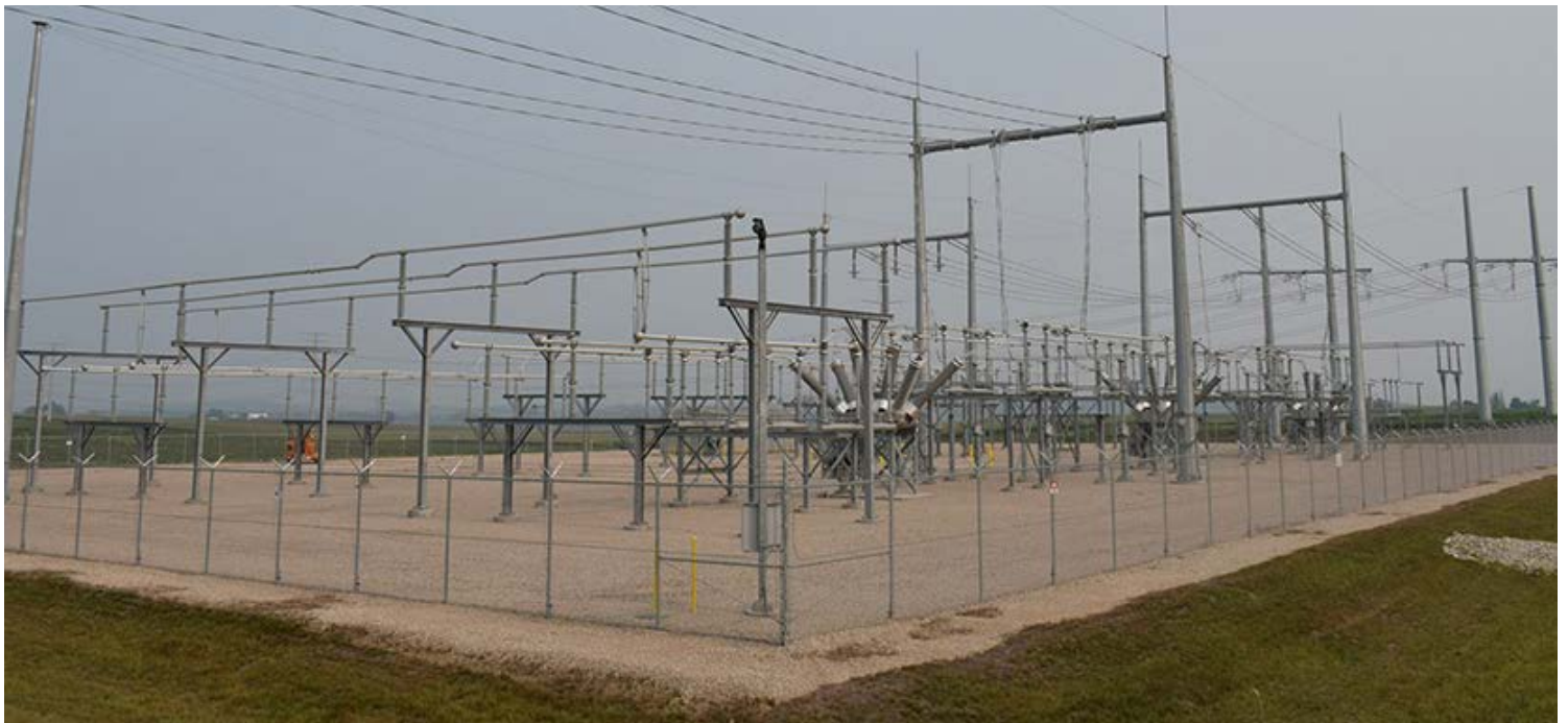
An ITC Midwest substation near Cedar Rapids, Iowa | ITC Midwest
