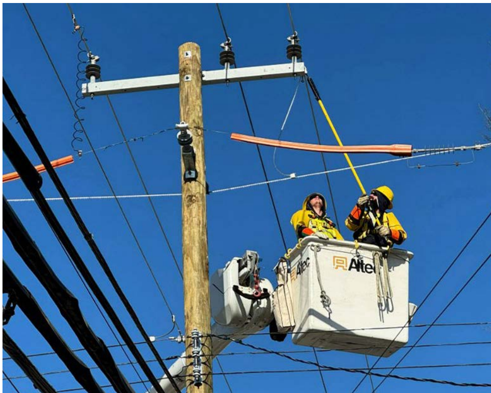
A DTE crew performs grid stability work in Wayne, Mich., in December. The Michigan utility is in line for billions in federal loan guarantees. | DTE
