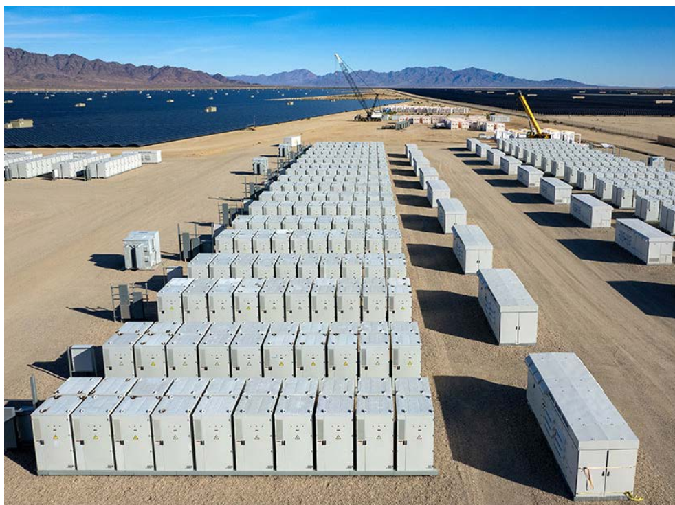
Rows of battery energy storage units are shown at the Desert Sunlight Solar Farm in Desert Center, Calif. | Shutterstock
