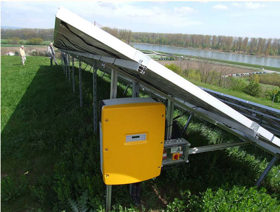
Inverter-based resource with electronic power converter | Claus Ableiter, CC BY-SA 3.0, via Wikimedia Commons
