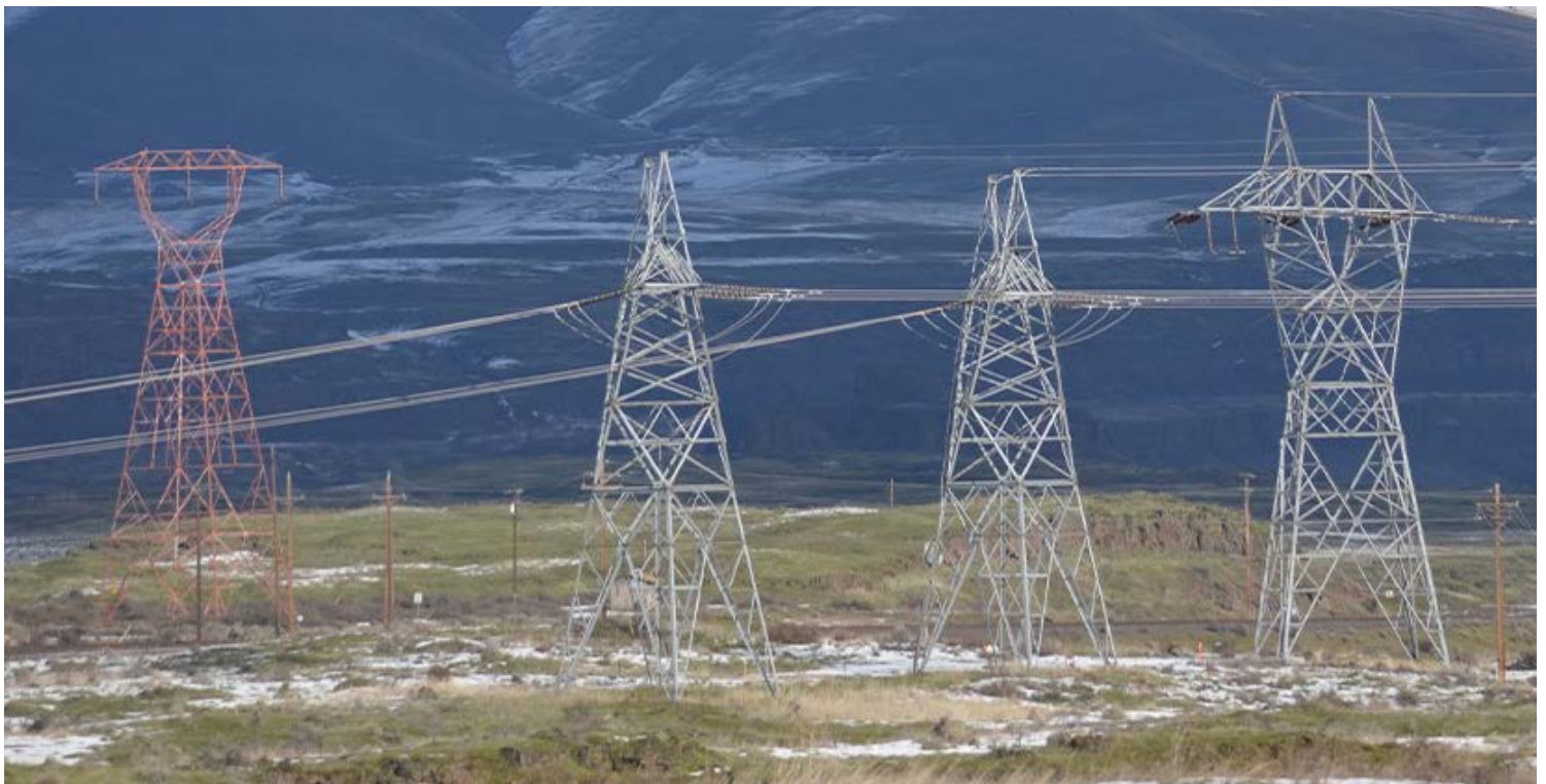
BPA transmission line in Oregon | © RTO Insider LLC
