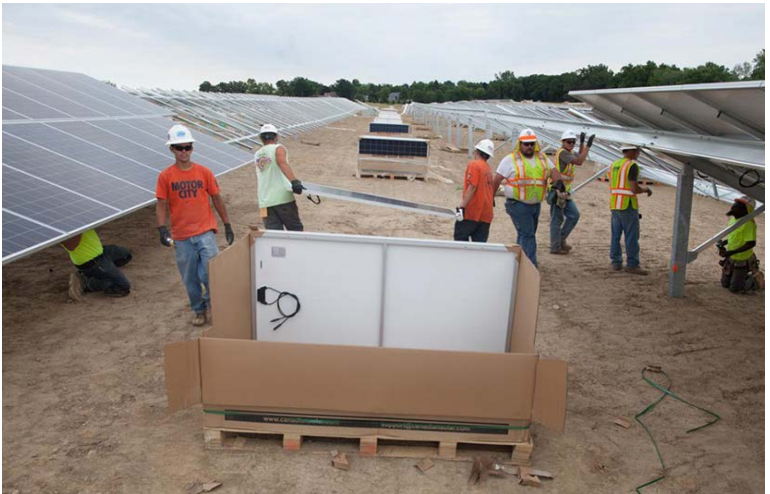
DTE Energy solar farm in Lapeer, Mich. under construction | J. Ranck Electric
