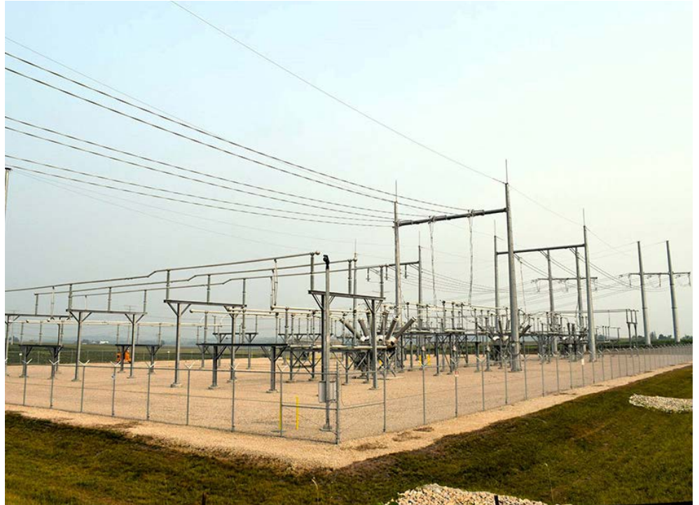
The Beverly-Morgan Valley Transmission Project in Iowa | ITC Midwest
